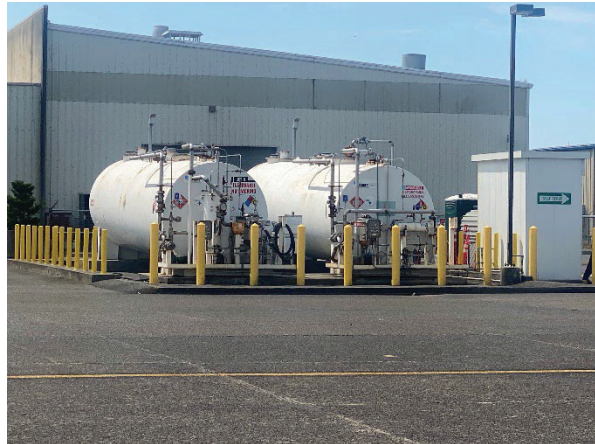
Figure 1-5: AST Aircraft Fuel Storage
