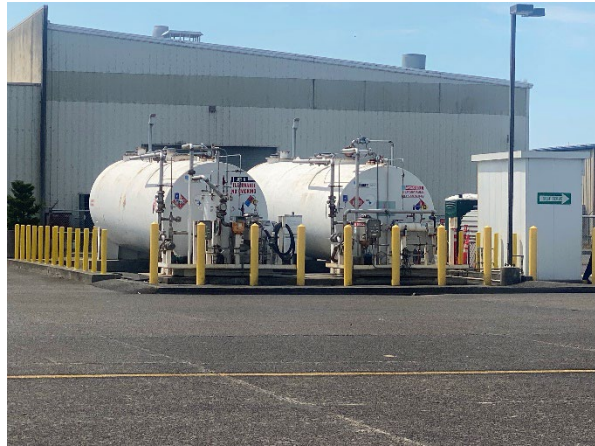
Figure 1-5: AST Aircraft Fuel Storage
