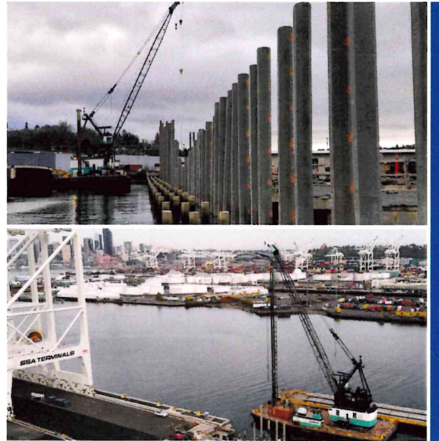
■ Terminal 5 Berth Modernization, Pier Strengthening & Berth Deepening - Port of Seattle Currently under contract
