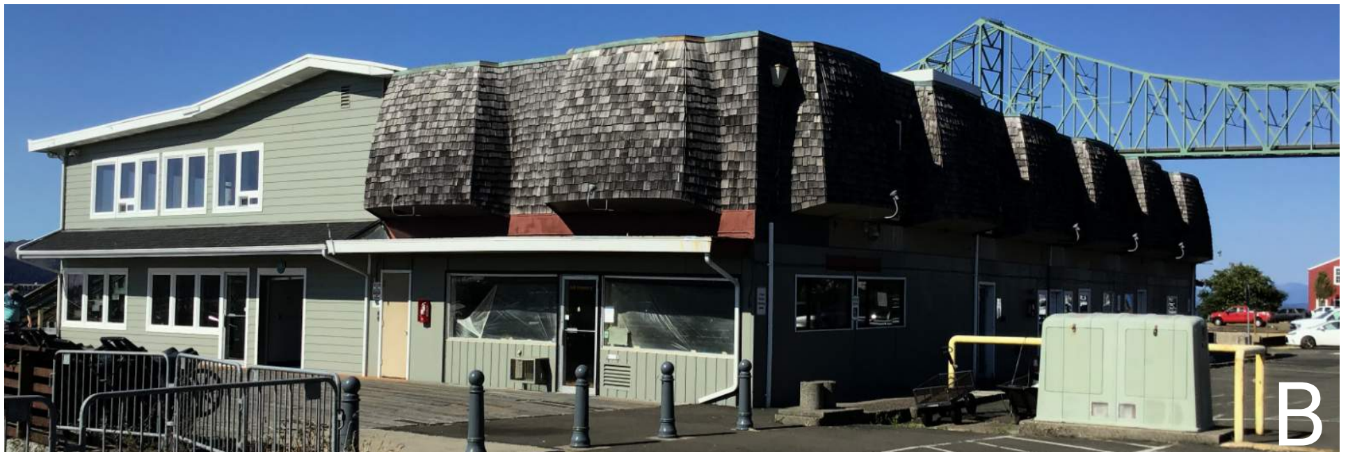
A: West elevation over the water with crane to unload fishing boats and equipment. B: South elevation (left) shows 1980s construction removed and rehabilitated, (right) is 1980s renovations showing deteriorated gutters, flashing, and drip edges that help to keep the building envelope dry.
